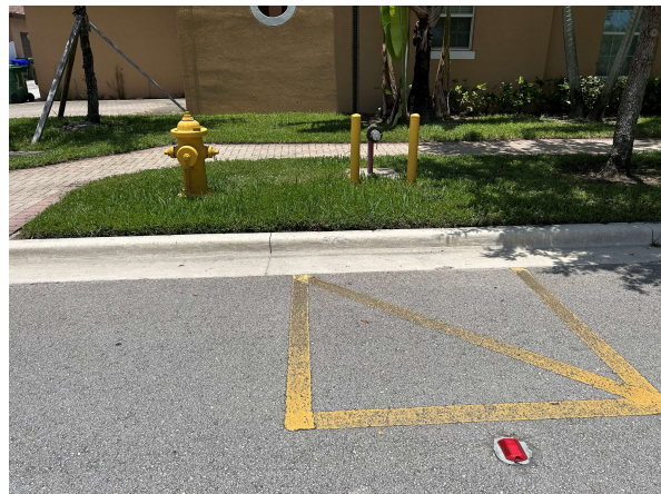
Phase II (FDC & Fire Hydrant) (18)
