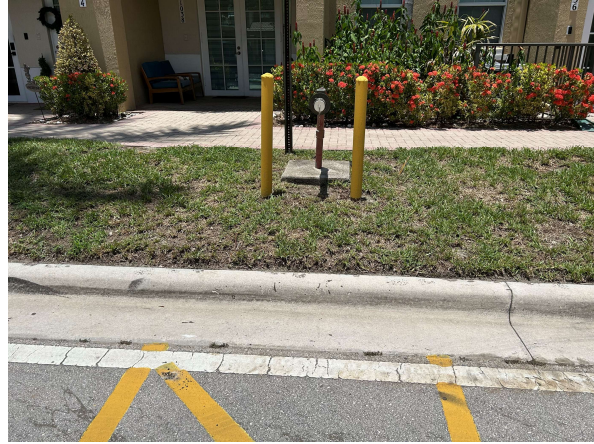
Phase II (Fire Department Connection) (16)
