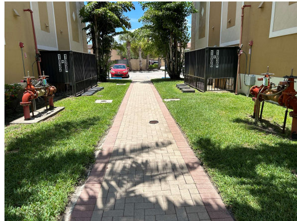
Phase II (Double Detector Check Valves) (14)
