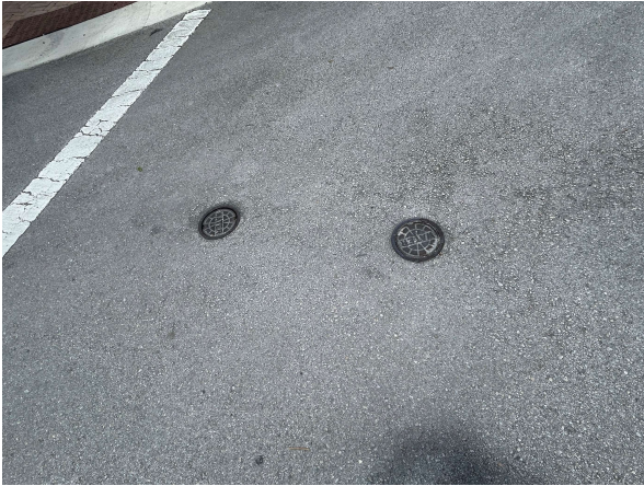
Phase I (Gate valves) (19)
