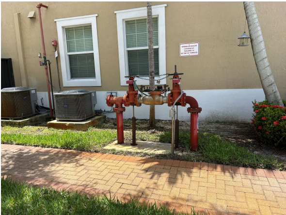
Phase I (Double Detector Check Valve) (13)
