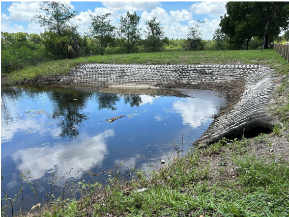
Wetland Conservation Area – Outfall Structure (9)
