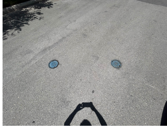
Phase II (Gate valves) (20)
