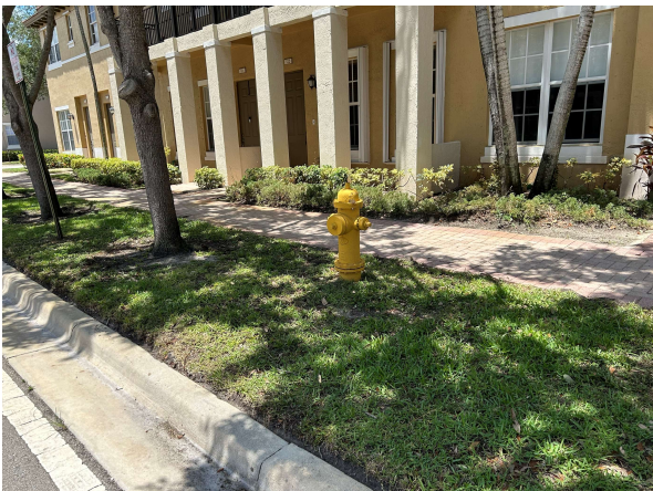
Phase I (Fire Hydrant) (17)
